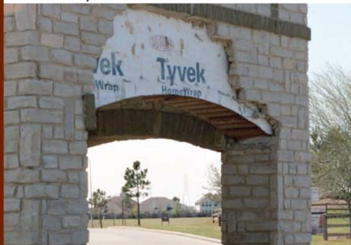
Consequences of not using fully installed arched lintel.
